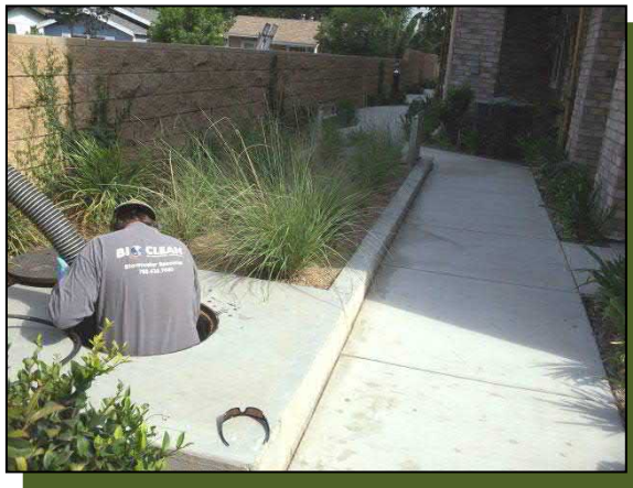
Vacuuming out of media filters.
